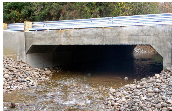
This 21 foot culvert was constructed in 2011 at an Unnamed Tributary to South Branch Big Creek on US 101 to replace a 6 foot culvert at milepost 102.14 north of Hoquiam for $1.1 million.
