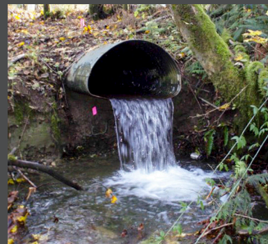
This 5 foot barrier culvert at Fortson Creek was replaced in 2012 with an 18 foot culvert at milepost 42.99 on SR 530 for $1.8 million.
