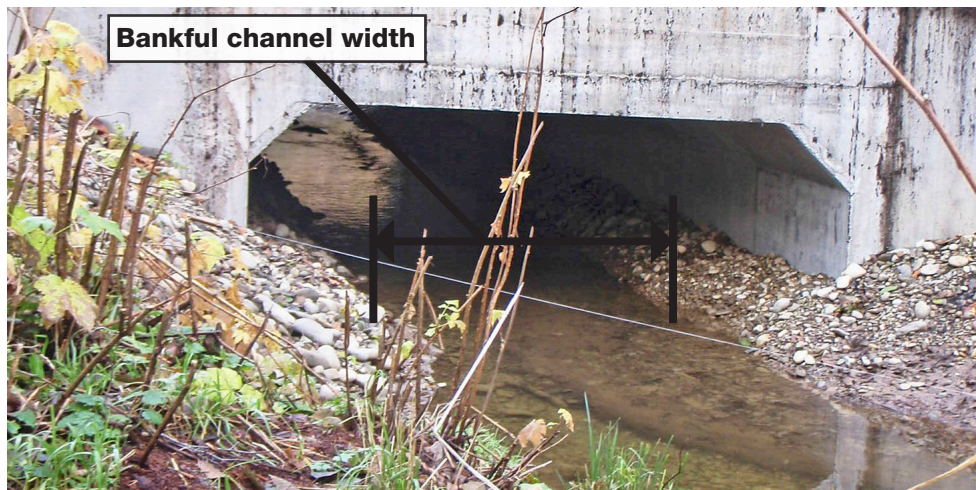
A 2.5 foot culvert was replaced with a 12 foot bottomless culvert. It was constructed in 2012 at an unnamed tributary to the Pysht River on SR 112 near Port Angeles for $1 million.
