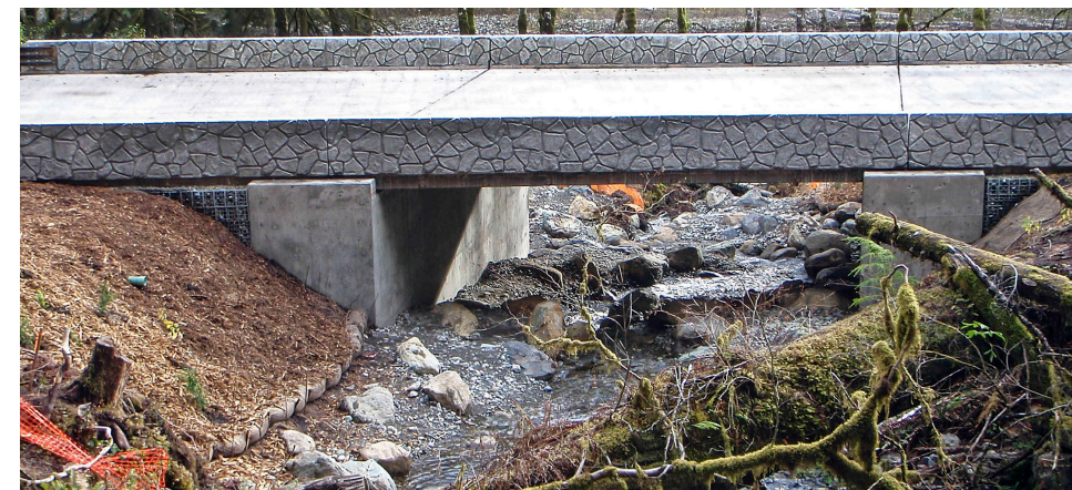
This 40 foot bridge was constructed in 2010 at Chain-Up Creek on SR 542 to replace a 5 foot barrier culvert at milepost 38.98 just east of Maple Falls for $1.3 million.
