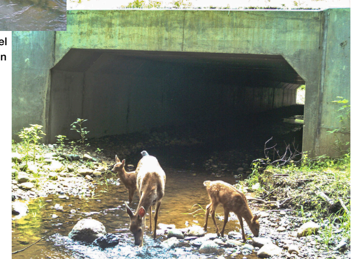
After – A 4-foot-round culvert was replaced with a stream simulation designed culvert that is 16 feet wide at Mosquito Creek on US 101 just southwest of Montesano. This new culvert provides habitat connectivity for deer and other animals as well as 2.2 miles of upstream habitat for fish for $1.4 million in 2009.
